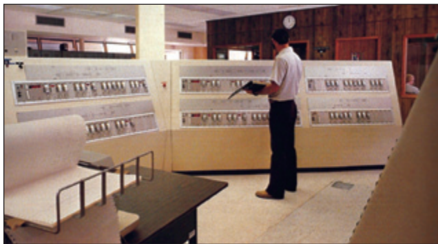
Figure 34. DYMAC monitors in an ammonia plant.
